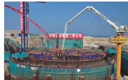
FUQING NUCLEAR POWER PLANT, CHINA 2008 Supply and supervision of PT for containment
